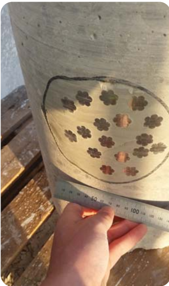
Core sample of void-free section showing cable tendons surrounded by Cable Grout
