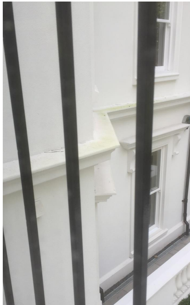
Profiles on the side wall showing both green algae and red lichen present but very limited mould black spot showing. These surfaces have very flat horizontal surfaces, allowing water to sit on them attracting the mould and algae spores to settle.
